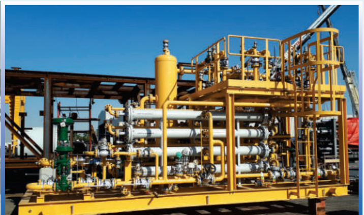
FUEL GAS CONDITIONING SKID
