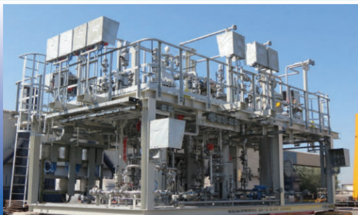
SEAL GAS CONDITIONING SKID
