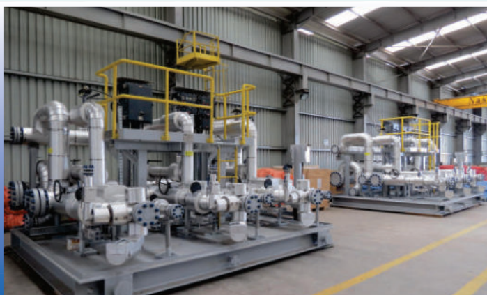
WELL MANIFOLD SKID
