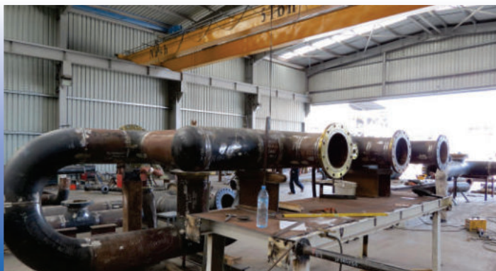
CARBON STEEL PIPING
