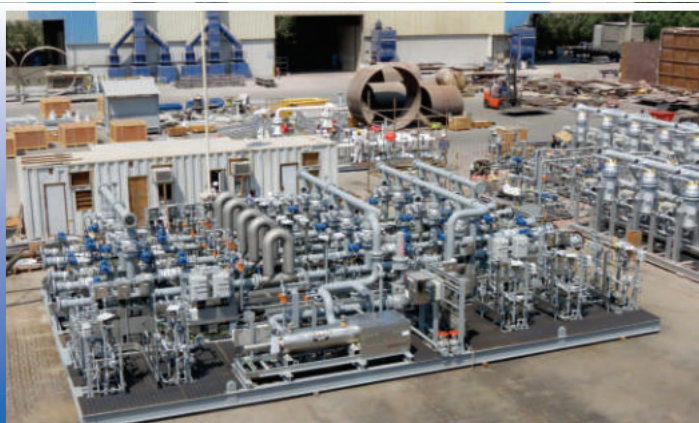
JETTY METERING & PROVER SKID
