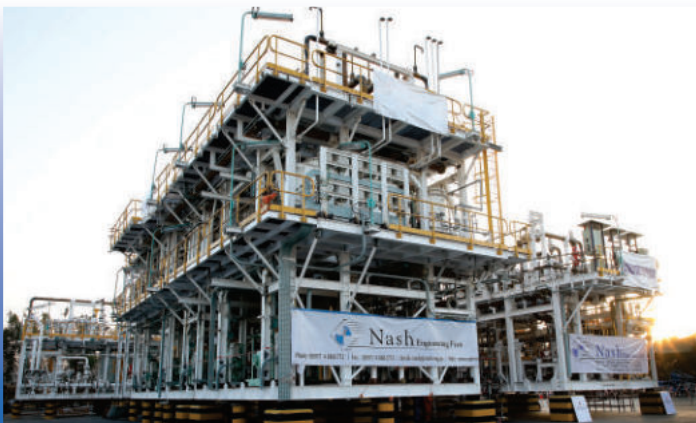
WATER INJECTION PACKAGE
