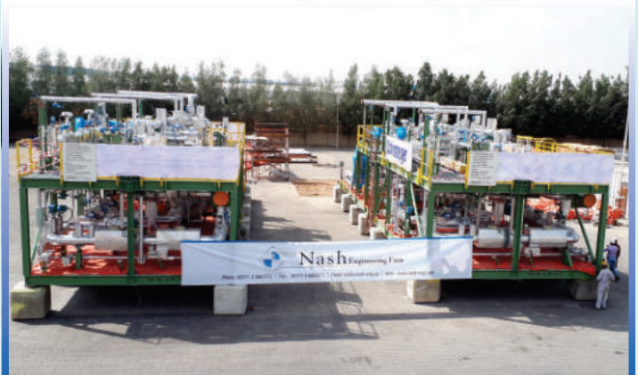
PRODUCED WATER TREATMENT PACKAGE
