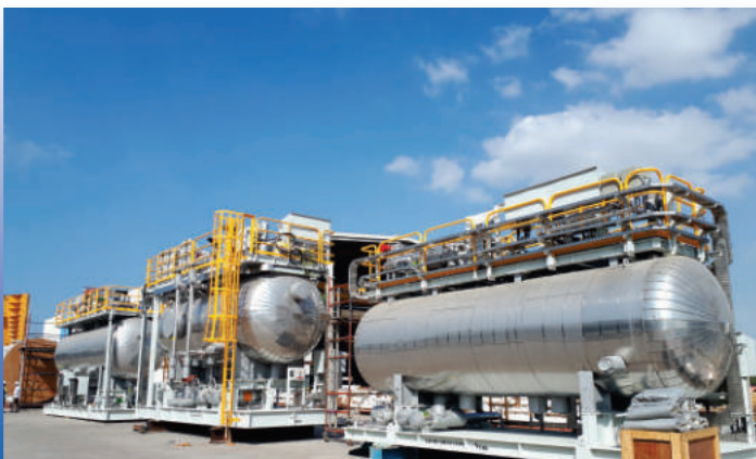
2 PHASE LP SEPARATOR SKID & BULLET TANK SKID
