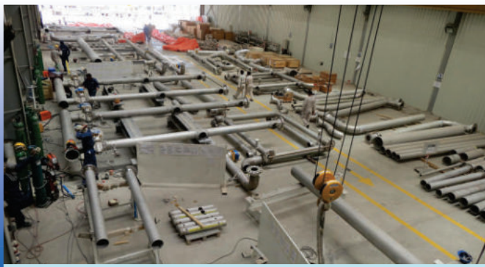
SUPER DUPLEX PIPING
