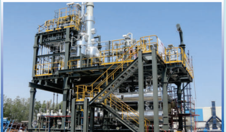
TEG SKID PACKAGE
